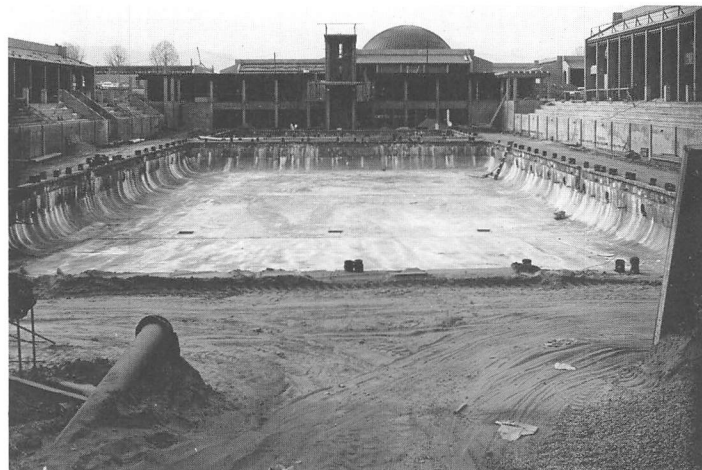
In 1966 as construction continues, the Minolta Planetarium dome looms in the background as De Anza's swimming pool complex takes shape. Photo from Foothill-De Anza District Archives.
