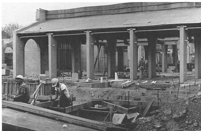
It took only 22 months from ground breaking to opening day for Cupertino's De Anza College to see the light of day. The college, celebrating its 25th anniversary this year, will be featured in a CHC exhibit this fall. Photo from Foothill-DeAnza District Archives.
